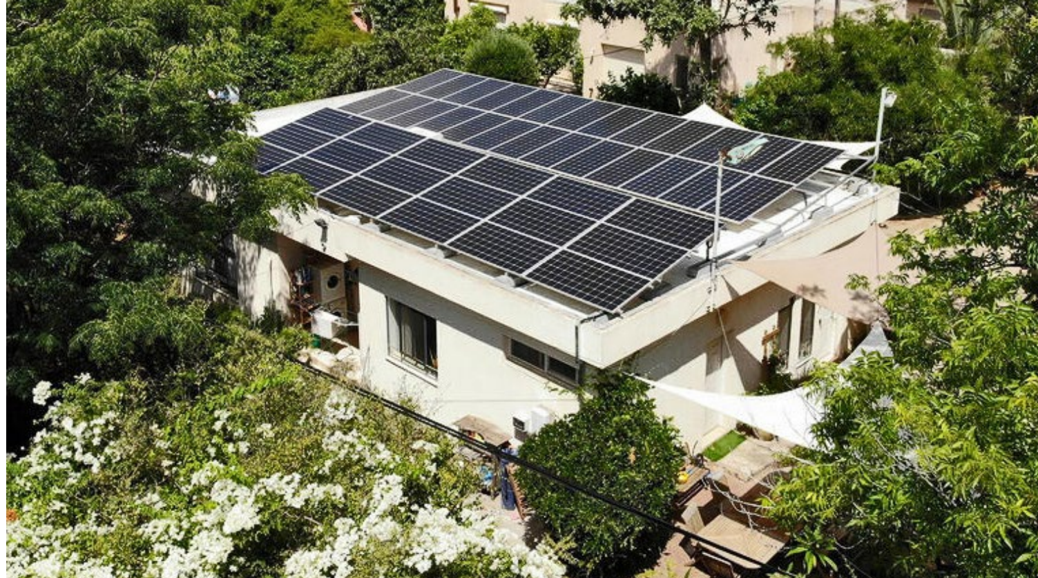
Solar Roofs (Credit: Volta Solar).
